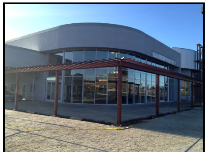
The trellis is up. It will provide support for vines which will serve to accent the outdoor courtyard to be used for social gatherings.
